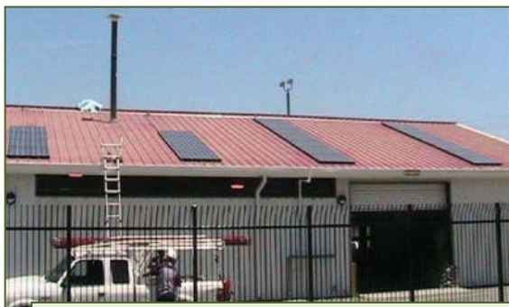
A photovoltaic system added to P&T operations at the Pemaco Superfund Site in Maywood, CA, contributes 5,900 kWh of electricity each year to high-vacuum dual-phase extraction of groundwater.
