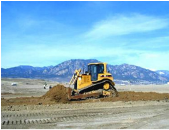
Evapotranspiration modeling led to a design and construction strategy employing thin (1-foot) lifts to achieve soil texture uniformity and to optimize dry bulk density of the landfill cover.
