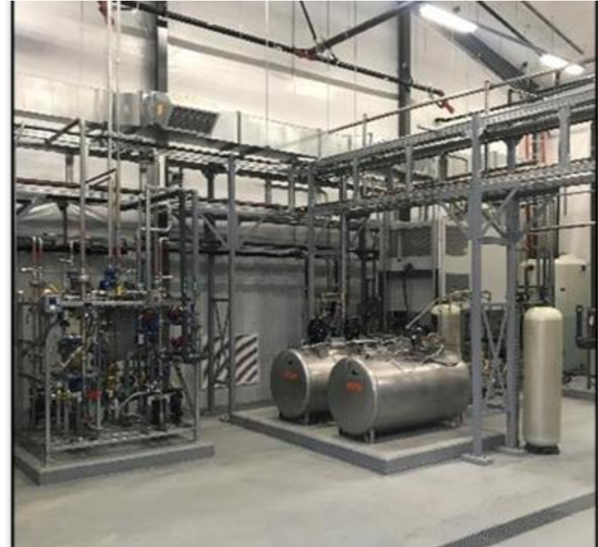
PFAS-1. Figure 15-14. Resin regeneration system. Source: Steve Woodard, ECT2, and Nathan Hagelin, Wood Group, PLC (WSP). Used with permission
