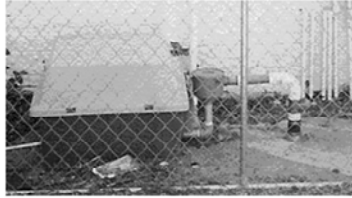
Figure 6-1. Small-scale soil vapor extraction (SVE) system designed to address the source of vapors. Photo Source: Vapor Mitigation Sciences, LLC.
