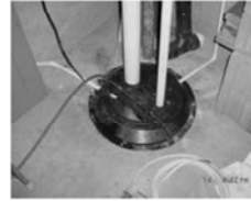
Figure J-4. Passive sump mitigation system. Photo Source: Kansas Dept. of Health and Environment
