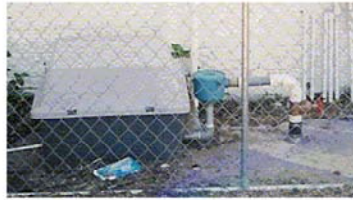
Figure 6-1. Small-scale soil vapor extraction (SVE) system designed to address the source of vapors. Photo Source: Vapor Mitigation Sciences, LLC.
