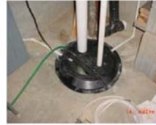
Figure J-4. Passive sump mitigation system. Photo Source: Kansas Dept. of Health and Environment
