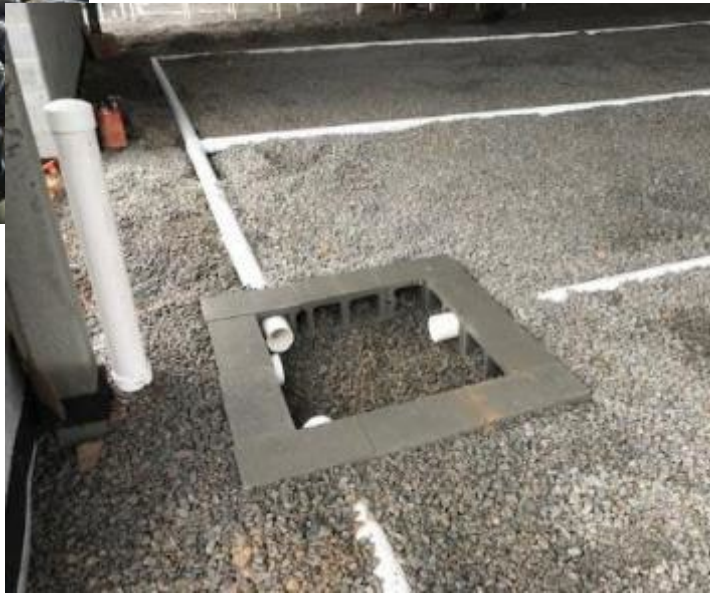
Passive Sub-Slab Venting (SSV) Systems
