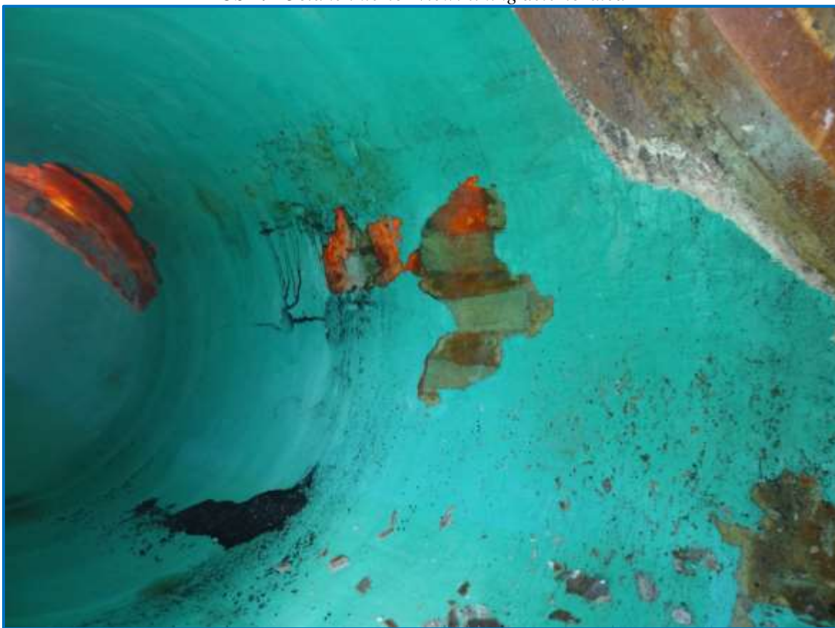
UST 92Octane interior view: lining deteriorated
