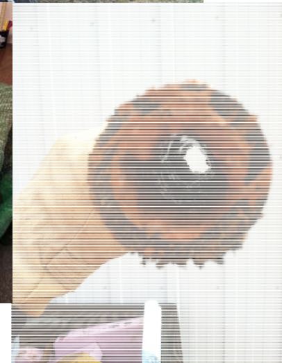
Iron Fouling of Process Pipes
