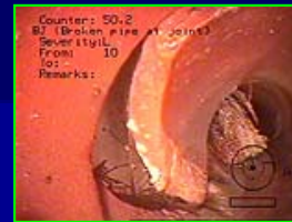
Broken and displaced pipe
