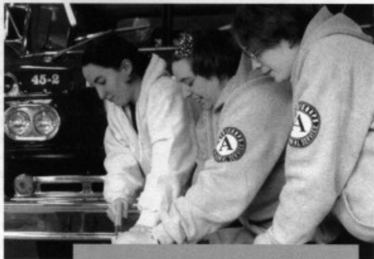
AmeriCorps volunteers Dana Serovy, Carla Ruddock, and Mary Beth King work together to construct a large planter box at a building day in Vintondale, Pa. The boxes are to be used in the new AMDCART park.
