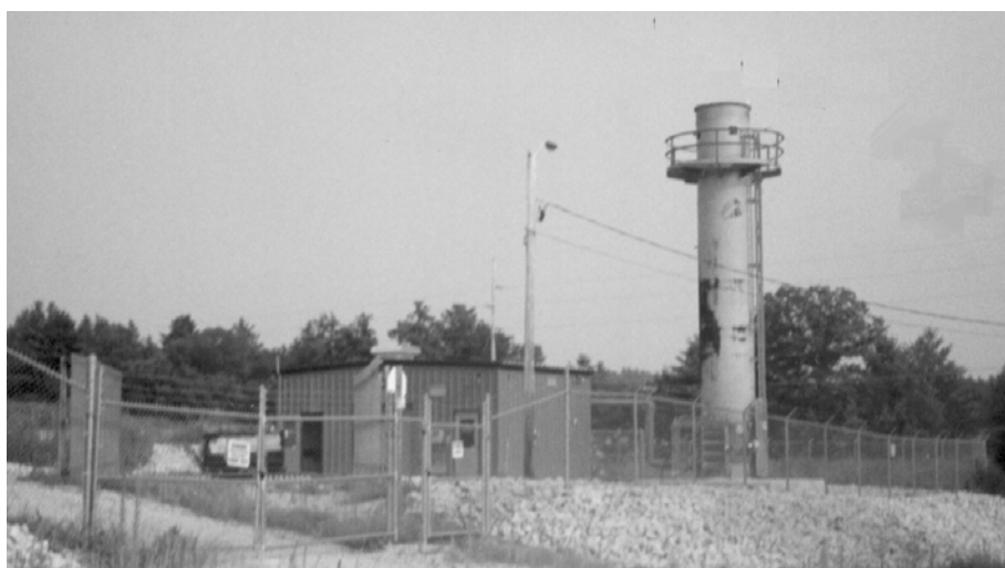
Figure 5-7. Enclosed Ground Flare and Blower Station.
