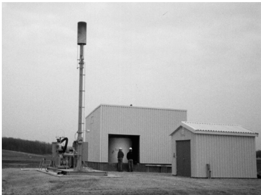
Figure 5-6. Skid-Mounted Open Flare and Blower Station.
