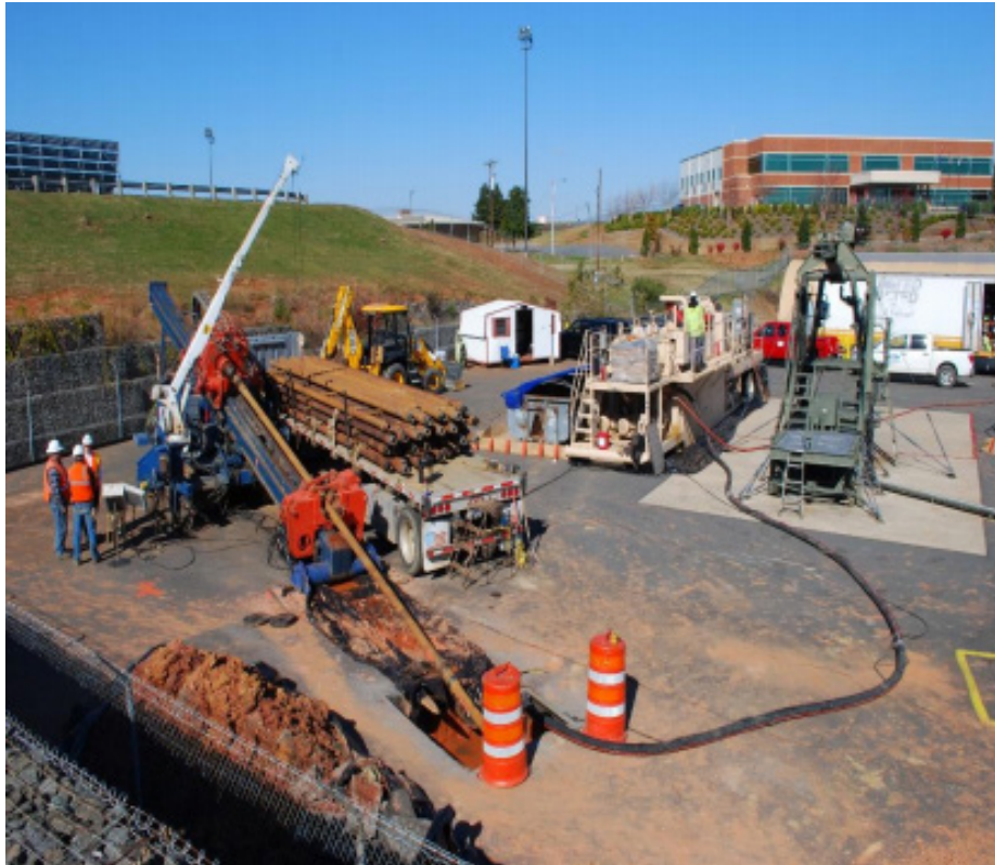
(Top photo reprinted from Directed Technologies Drilling, Inc. website (2015) with permission of Directed Technologies Drilling, Inc. Bottom photo reprinted from Horizontal Environmental Drilling 101 – An Introduction to the Means and Methods for Horizontal Environmental Well Installation (2014) by David Bardsley with permission of Directed Technologies Drilling, Inc.)
