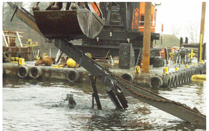
Material Recycling: Timber and steel connected to a pier along Curtis Creek were salvaged during sediment dredging and sold to local recycling companies.
