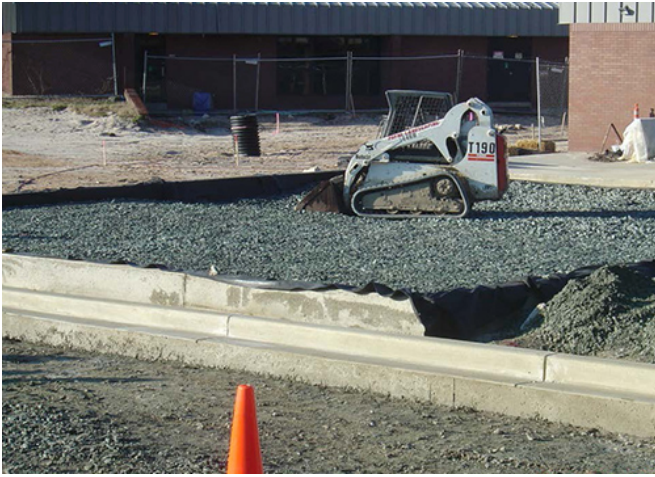
Drainage Control: Management of drainage in the former salvage lot involved integration of conventional and green infrastructure practices such as installing a subsurface, engineered drainage system below permeable pavement.
