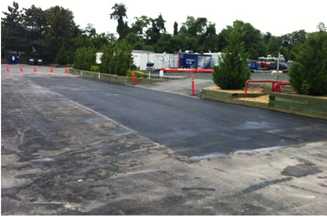
Erosion Control: An eroded embankment between the former salvage lot and the former burn pit was stabilized by installing wood frames filled with deep-rooted plants and surface material capable of capturing and retaining stormwater, thereby reducing runoff.
