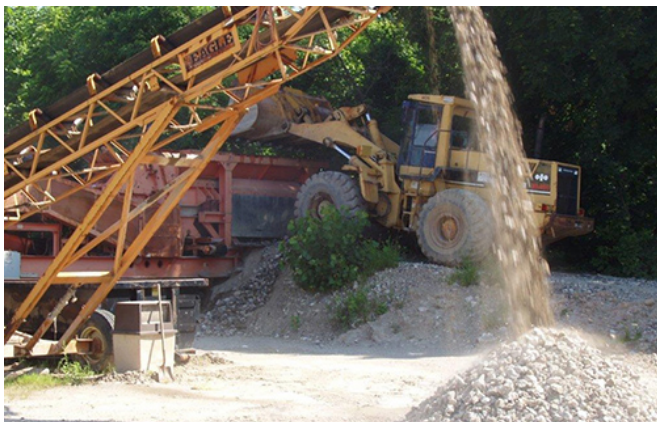
Onsite Reuse of Material: Nearly 2,300 cubic yards of concrete was salvaged during onsite demolition and re-used onsite as infill for excavated areas.
