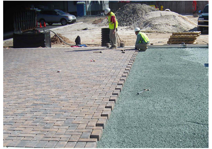
Permeable Pavement: The permeable pavement in the former salvage lot consists of brick pavers set on a base of rock mixed with sand. Joints between the pavers were filled with additional sand to allow water to percolate downward.
