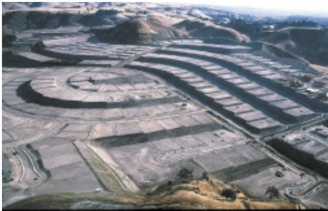
Figure 4. “Earthworks for Hillside Housing.” Near Los Angeles, Calif. Photograph by Alex S. MacLean (Corner and MacLean, 1996, p. 67). Courtesy of Yale University Press, New Haven, Conn.
