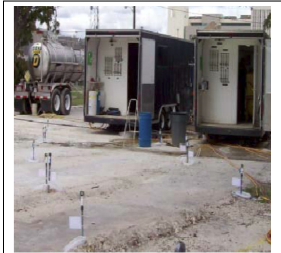
Figure 2. Oxidant Tanker and Control Trailers
