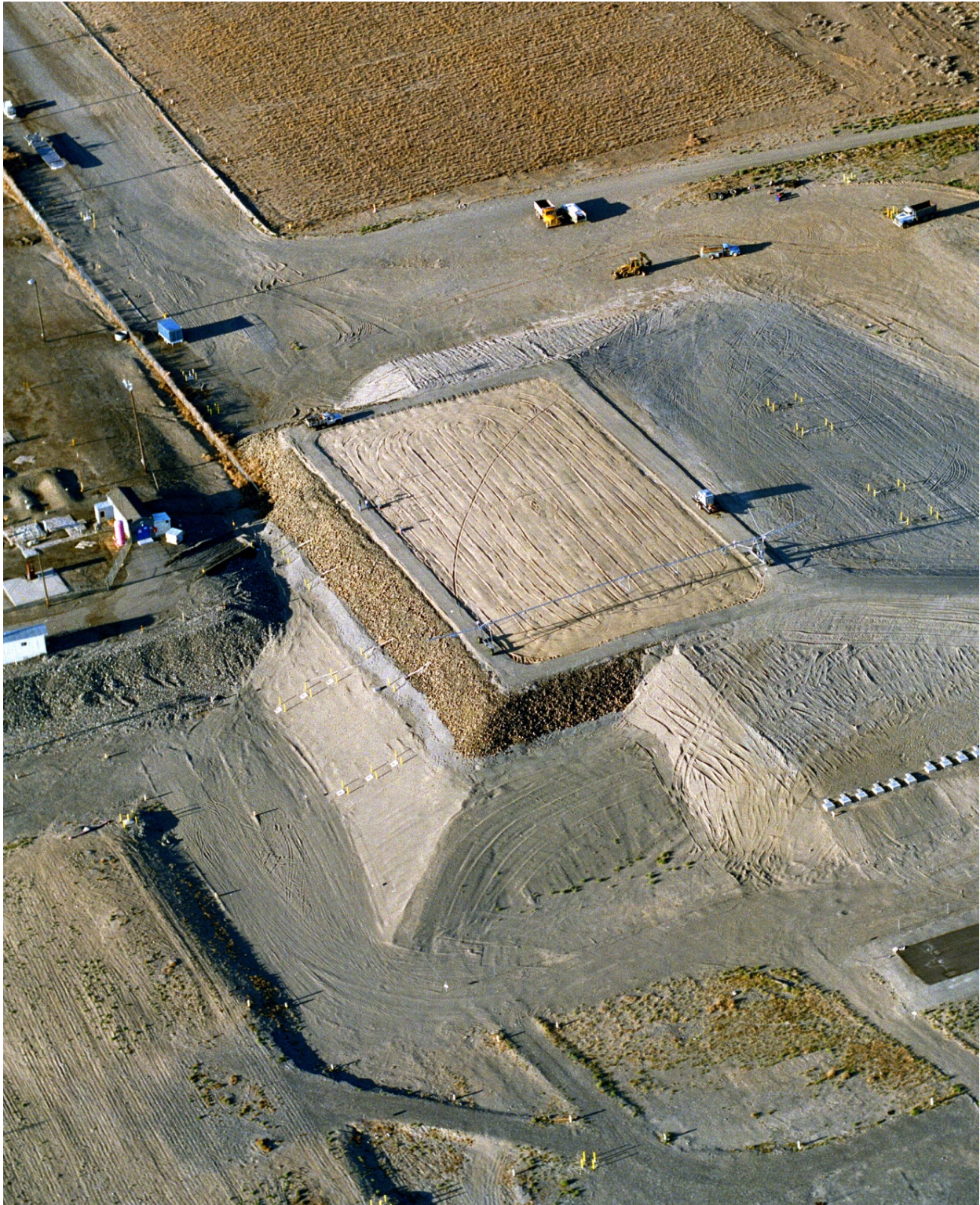
Figure O.1. The Prototype Hanford Barrier on August 9, 1994 (southwest-facing view). The two side-slope configurations and drainage monitoring system are to the north.
