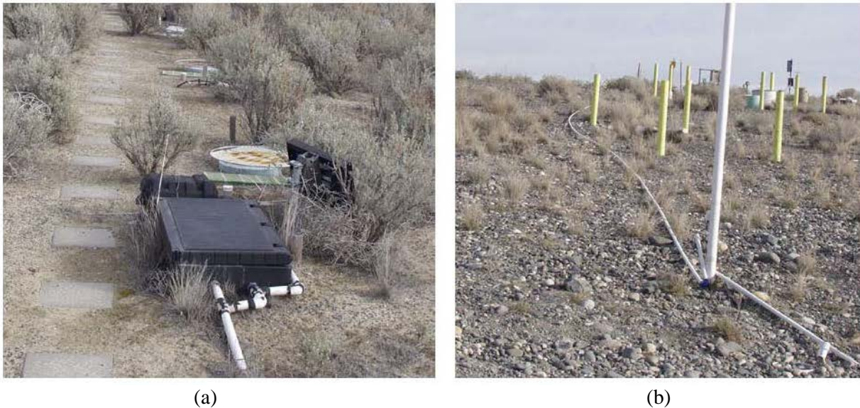
Figure B.10. Photographs of the barrier surface and gravel side slope showing examples of monitoring infrastructure, (a) instrument boxes containing dataloggers, and (b) conduits carrying communication cables for instruments, that needed protection during the controlled fire.
