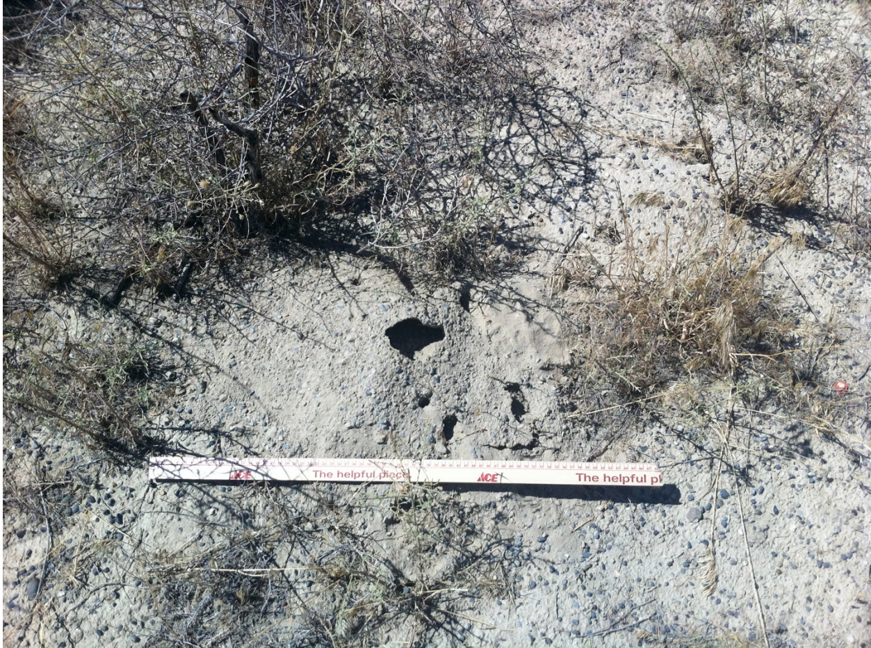
Figure L.6. Large Animal Hole with Five Nearby Holes on the Burned Section of the Barrier Surface.
