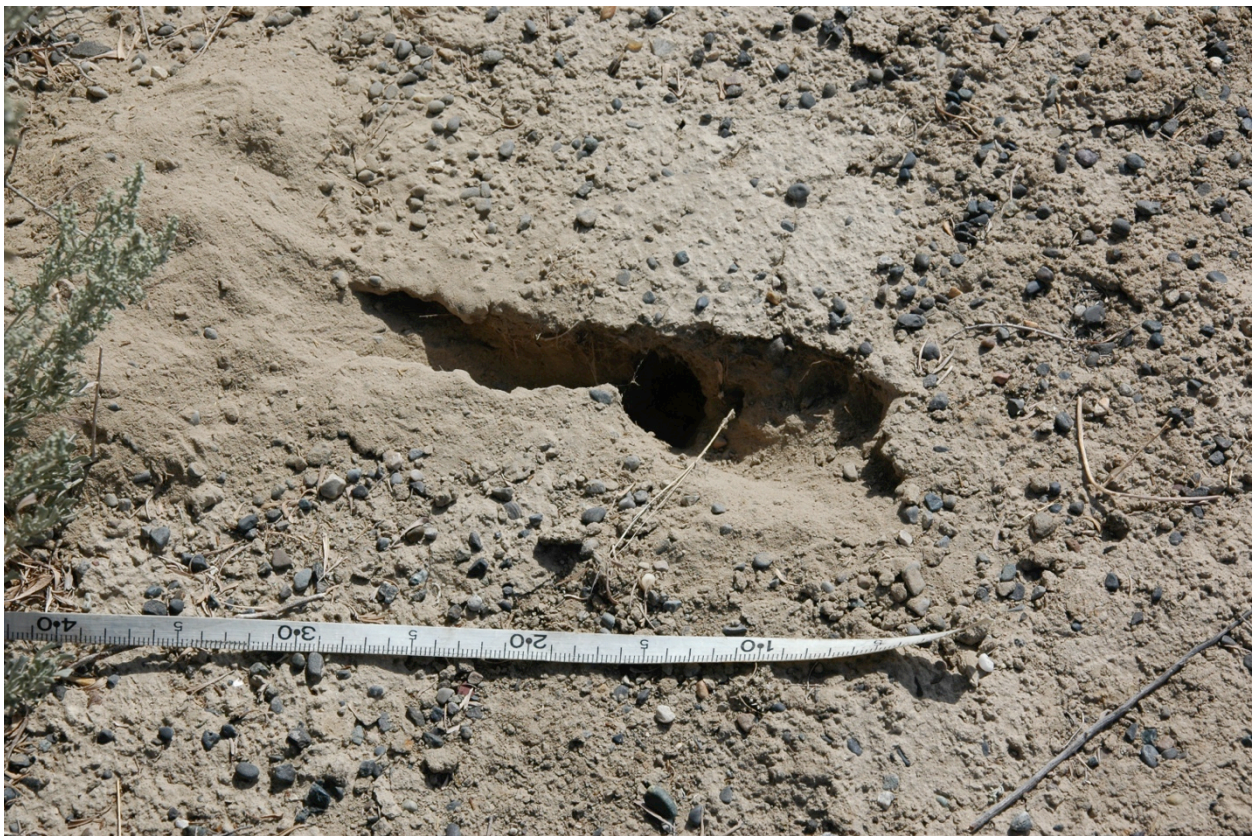
Figure L.2. Small Animal Hole on the Barrier Surface. Note recent digging activity in the upper left hand corner.
