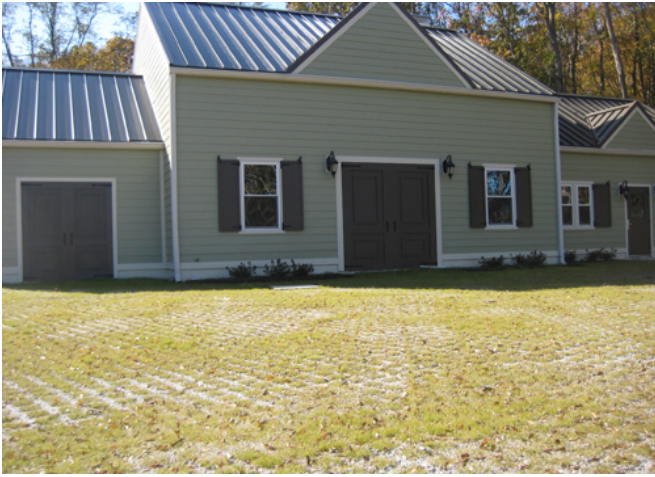
Pervious Pavement: During design of the offsite treatment plant, the Port Jefferson Beautification Committee worked with EPA Region 2 to develop landscape plans that included a "living driveway" of pervious pavement. The paving product is manufactured from materials sourced approximately 25 miles from the LAI site.
