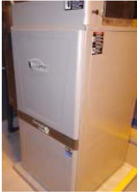
Heat Exchanger: Heat from groundwater entering each exchange unit is transferred to the air by way of metal coils inside the unit.
